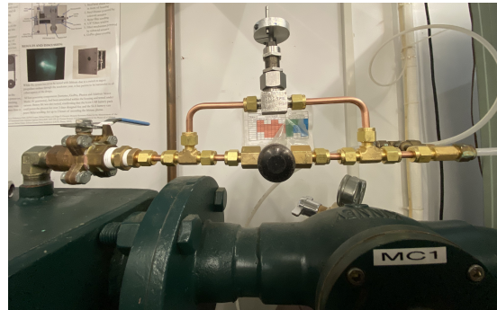
Figure 4.12: Parallel piping system installed between the argon cylinder and the glovebox.
